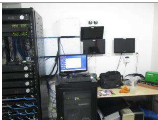
Central de controle
